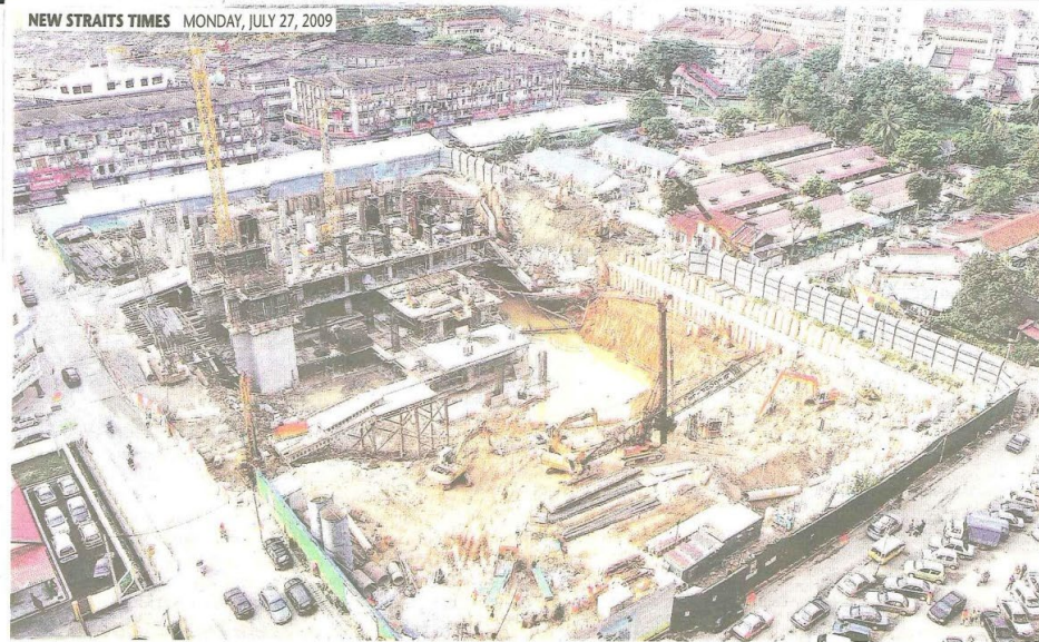
There is development on one side of the Lorong Gelugor cave-in, which occurred near the houses with blue roofs. — NST pictures by Ahmad Irham Mohd Noor
