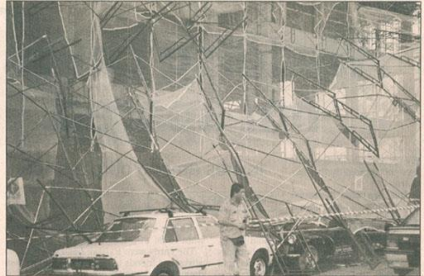
ABOVE: The fallen structure in Puchong
