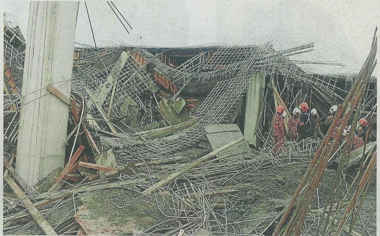
Deadly development: Fire Department personnel inspecting the scene of the deadly collapse in Ulu Tiram, Johor.
