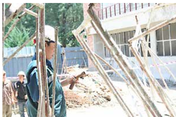
Figure 8: Proper inspection can identify defective components and formwork and falsework are used according to the design assumptions and limitations.
