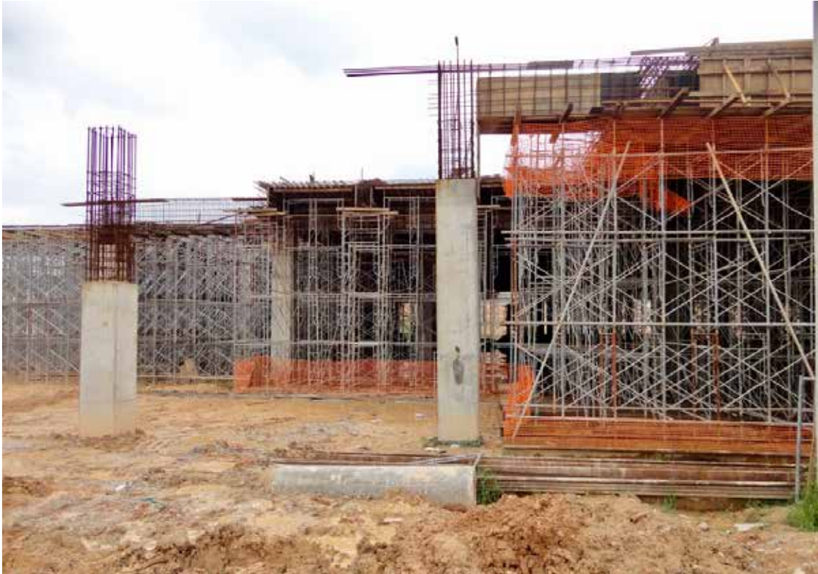
Figure 2: Formwork and falsework are “engineering solutions” used to support wet concrete to form permanent structures (for example, reinforced concrete columns, beams and slabs) during construction.
