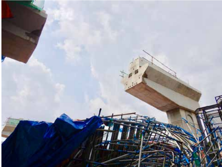
Figure 1: In many investigations of formwork and falsework collapsed, the authors found that there was insufficient consideration given to the safety management of these structures.
