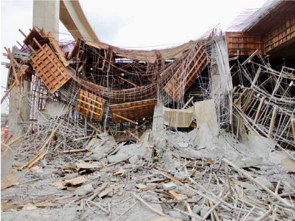
Figure 4: The safe work procedure prepared by the contractor and the PEPC must be fail-safe to ensure that workers are not at risk of injury while working with the formwork and falsework.
