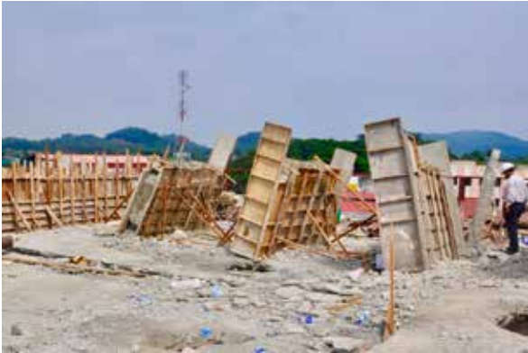
Figure 9: The formwork and falsework structure need to be tied and braced to accommodate lateral forces.
