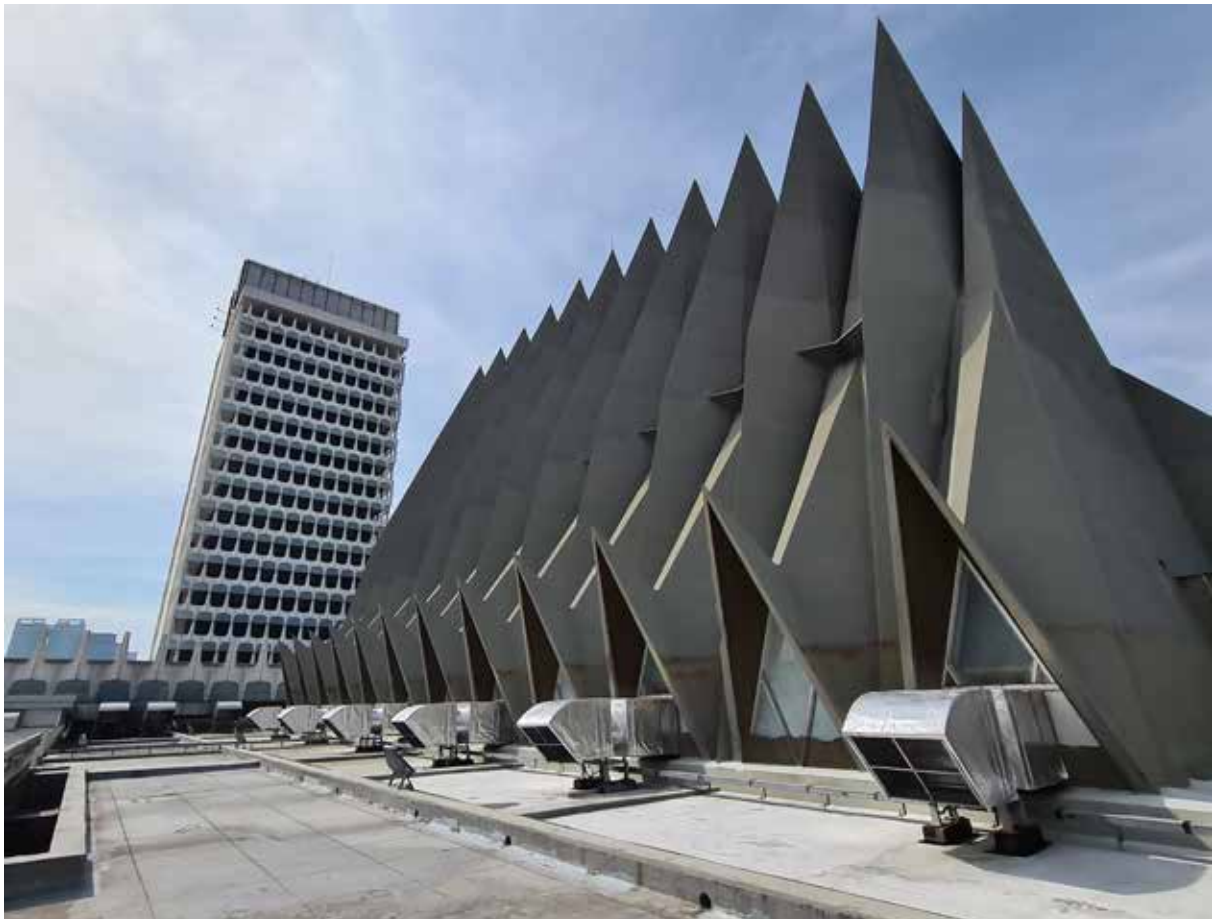
Figure 14: View of the present lower rooftop after waterproofing repairs and omitting the pool system
