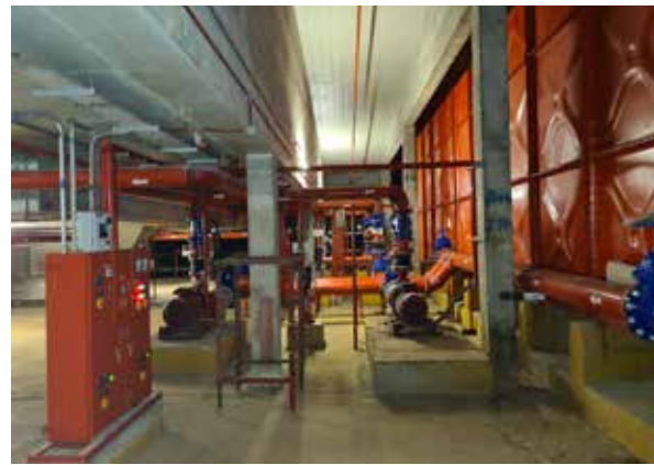
Figure 8: The new mechanical firefighting water tanks
