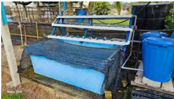
Figure 1: AquaBAE system installed at the Kebun Komuniti Suria Residences.
